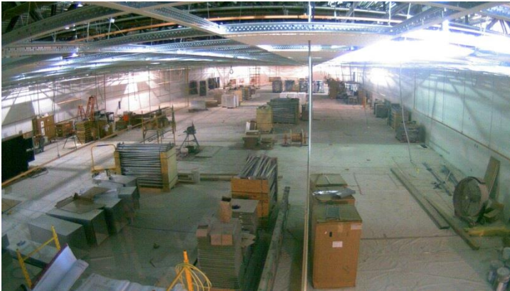
Illinois Petascale Computing Facility
